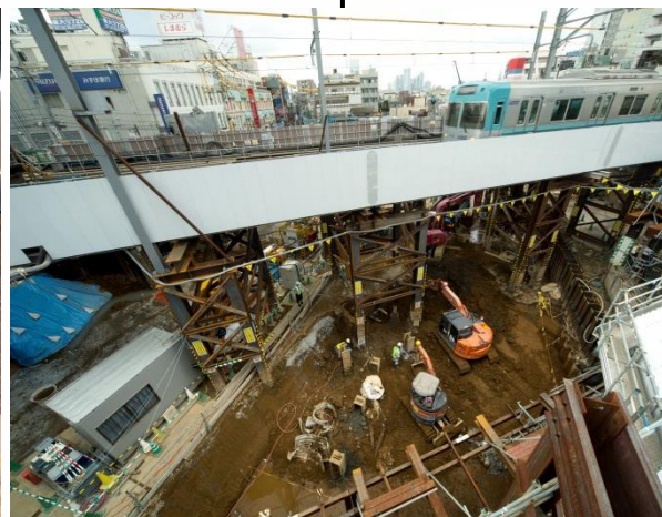
京王井の頭線橋梁架け替え工事 Keio Inokashira Line bridge replacement construction
